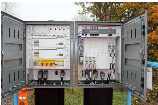
Fig. 9: Object controller cabinet
