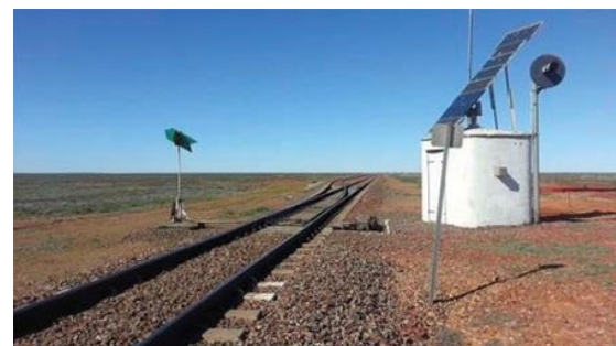
Fig. 10: Power supply in remote areas is ensured by solar panels
