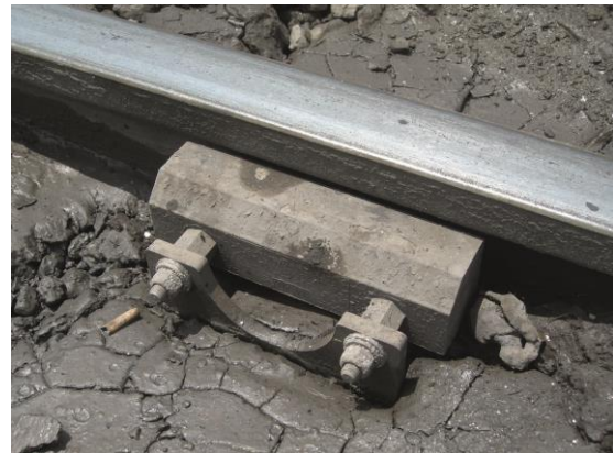
Fig. 4: Frauscher Wheel Sensor after flooding
